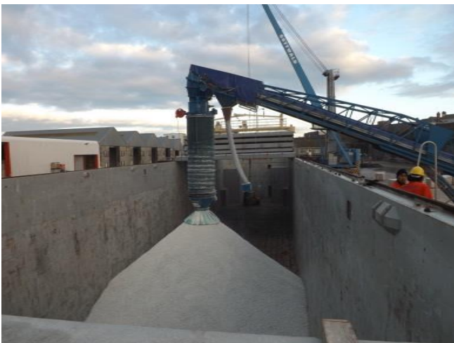
The Ship Loading Chute is used to load kaolin and is capable of loading at rates of up to 500tph
