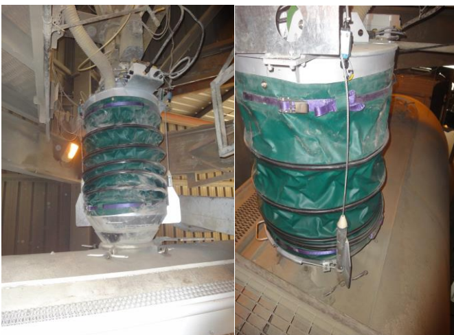
The Tanker Loading Chute is used to load cement and is capable of loading at rates of up to 150tph
