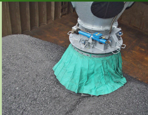
Above: Cleveland Cascades Cascade Shiploader – Petroleum Coke, Immingham, UK.
