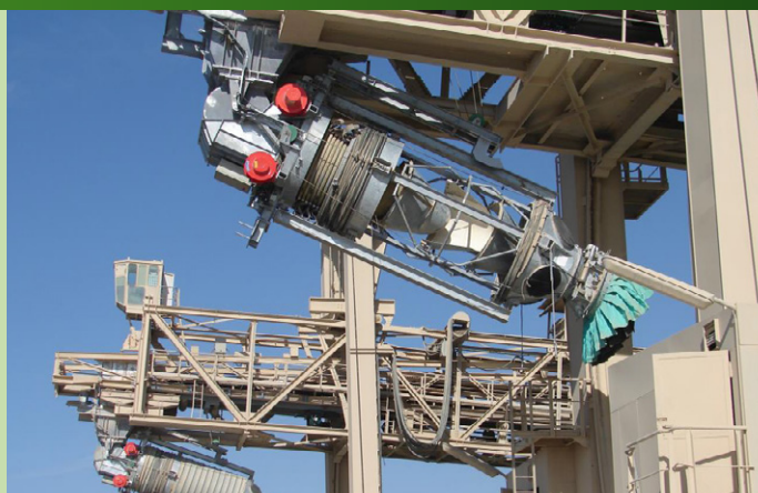
Above left: Cleveland Cascades Cascade Shiploader – Phosphate, Port of Aqaba, Jordan Above right: Cleveland Cascades Ship Loader - Phosphates, Christmas Island
