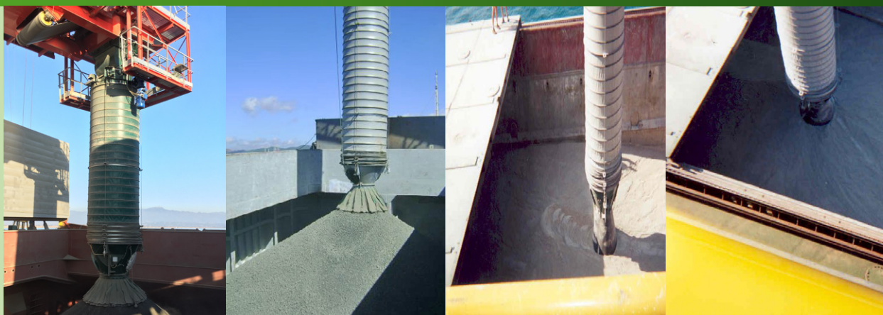
Left to right: Cleveland Cascades Ship Loader - Clinker, Turkey Cleveland Cascades Cascade Shiploader - Loading Cement Clinker. | Cement Powder.
