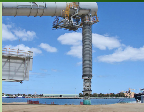
Above: Cleveland Cascades Cascade Shiploader – Alumina, Bunbury Port, Australia.
